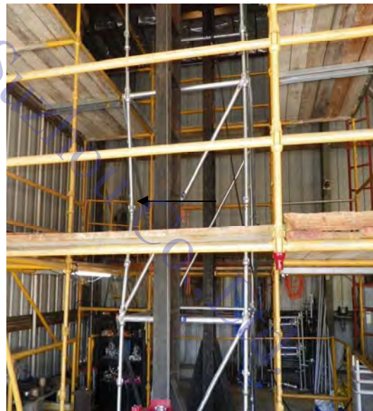
Typical deflection of leg at failure
